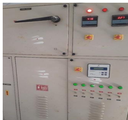
Figure 6. A 50 kVA capacitor bank
